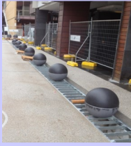
Steampacket Place Geelong one of the demonstration projects designed using Sustainable Infrastructure Guidelines
